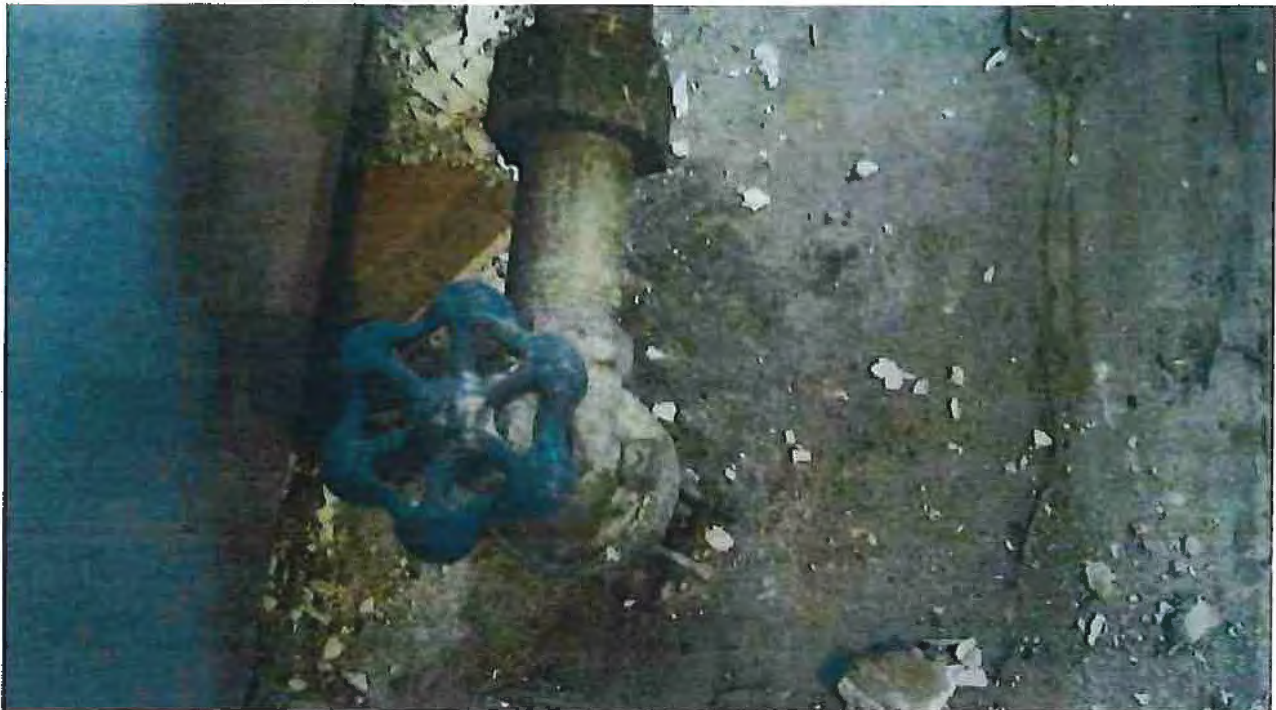
Figure 2 - Overhead View of Water Service Line Valve
